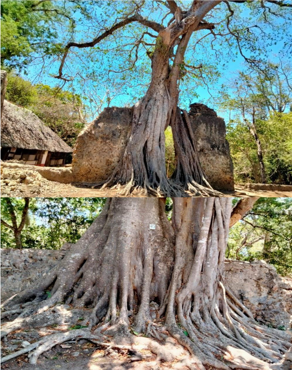
Plate 8: Section of Ruin engulfed by the fig Tree. Tree roots and plant stems dig in to the heritage causing eventual crumbling of the ruins at Gede
